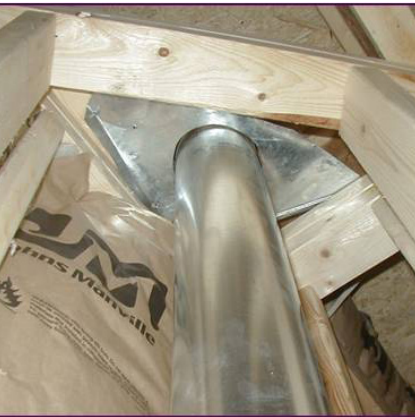
INCORRECT: Improperly capped chase
