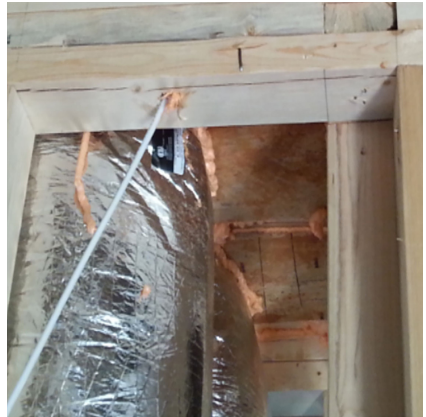
CORRECT: Capped chase properly sealed
