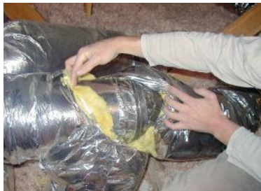
INCORRECT: No Mastic
