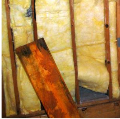
INCORRECT: Unfilled cavity
