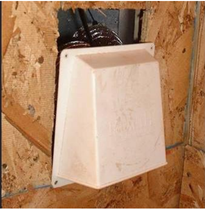
INCORRECT: Unsealed sheathing penetration
