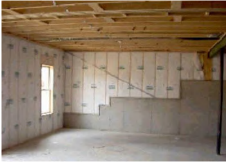
INCORRECT (CZ3-4): Insulation not on concrete portion of basement wall.
