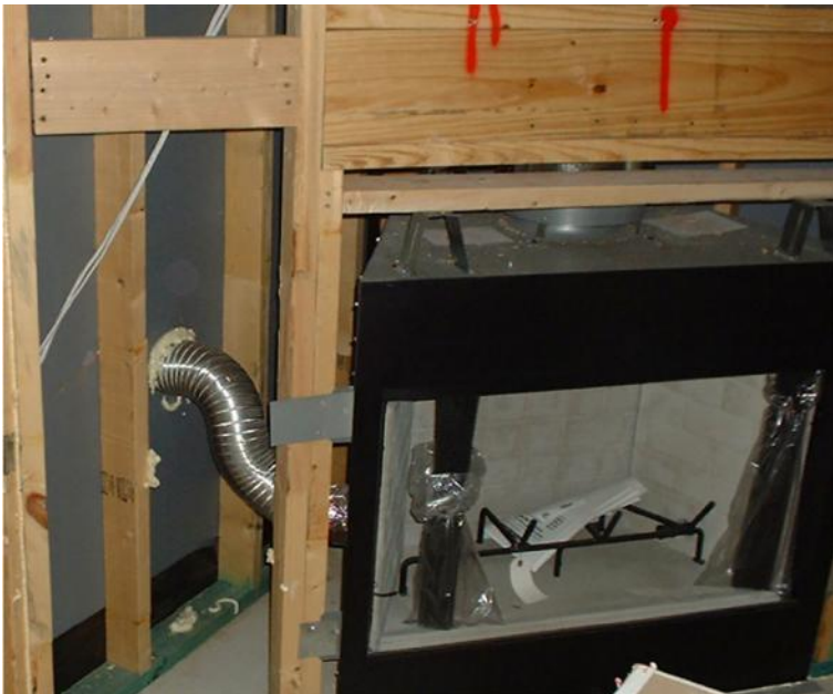
Wood-burning fireplace features dampered outdoor combustion air and tight-fitting flue damper.
