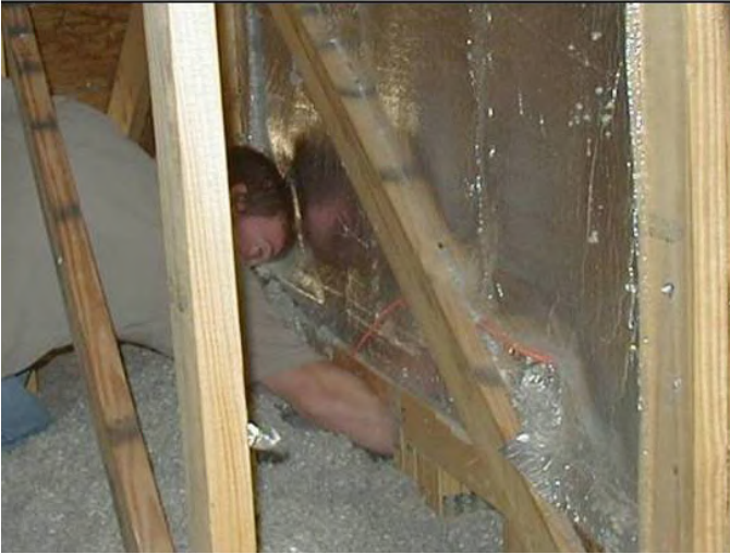
INCORRECT: Unblocked joist cavity. Inspector is reaching through the unblocked joist cavity revealing a significant pathway for unconditioned attic air into the building envelope.
