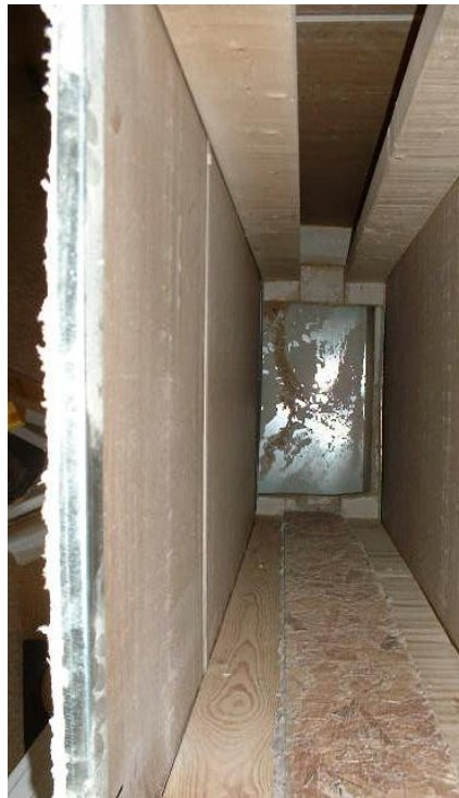
INCORRECT: Unlined cavity as plenum
