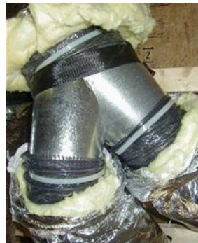
INCORRECT: UL-181 Tape without Mastic
