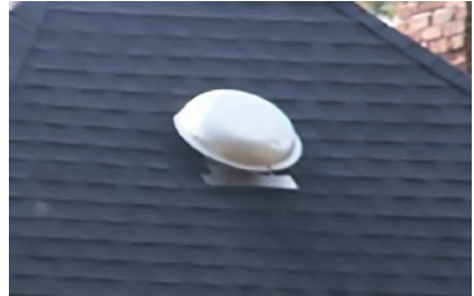
NOT ALLOWED: Grid-tied ventilator
