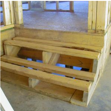
INCORRECT: Air bypass behind stairs
