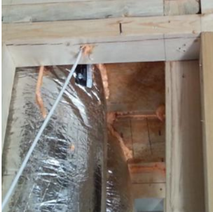
CORRECT: Capped chase properly sealed
