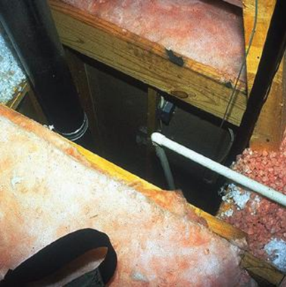
INCORRECT: Unsealed chase
