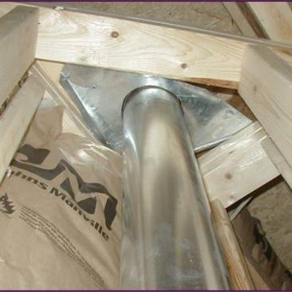
INCORRECT: Improperly capped chase
