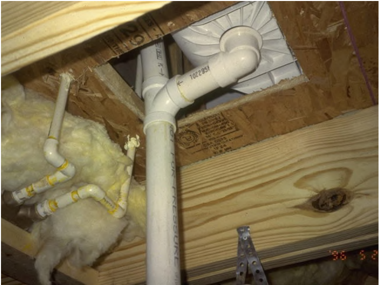
INCORRECT: Drain penetration open
