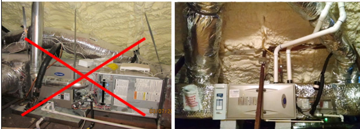
Figure 41: (Left) A poor decision - where will combustion air come from in this unvented attic assembly? (Right), a correct 2-pipe 95% AFUE furnace that is properly installed in this (retrofitted) unvented foamed attic (Lindsley attic). [Barcik photos]
