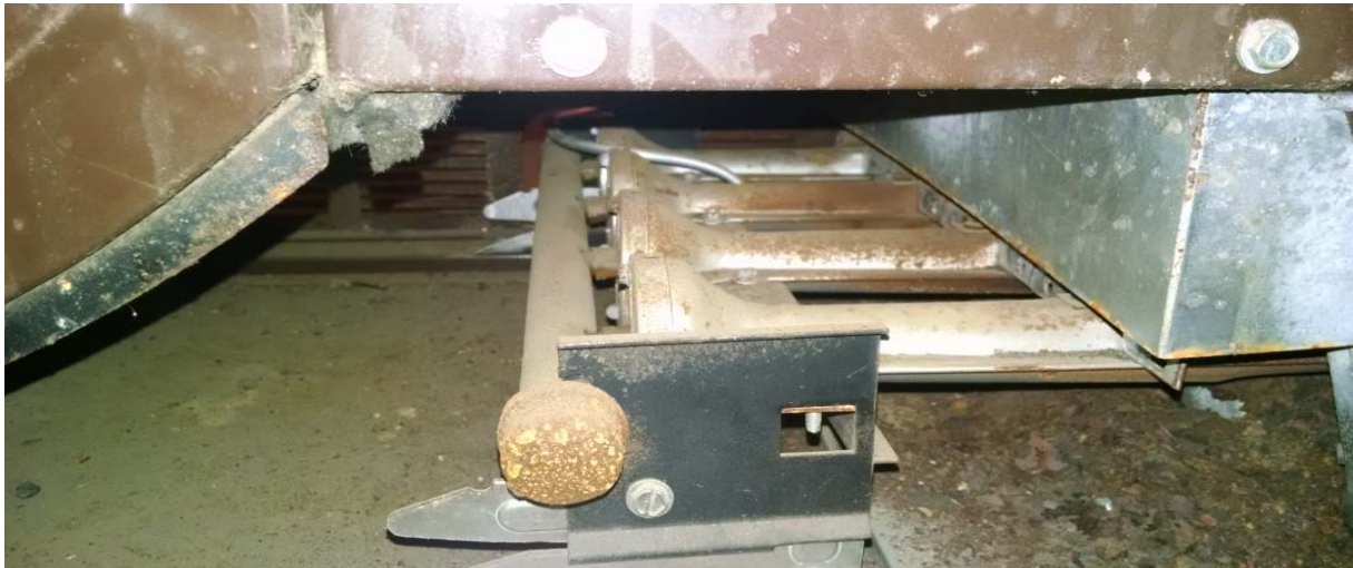
Figure 35: Four burner atmospheric furnace (historic building). [Barcik photo]
