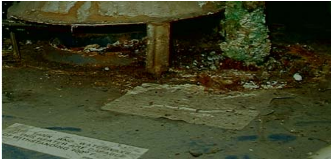
Figure 26: Extreme corrosion on draft diverter and on water line caused by condensation due to faulty drafting (WX1). [Barcik photo]
