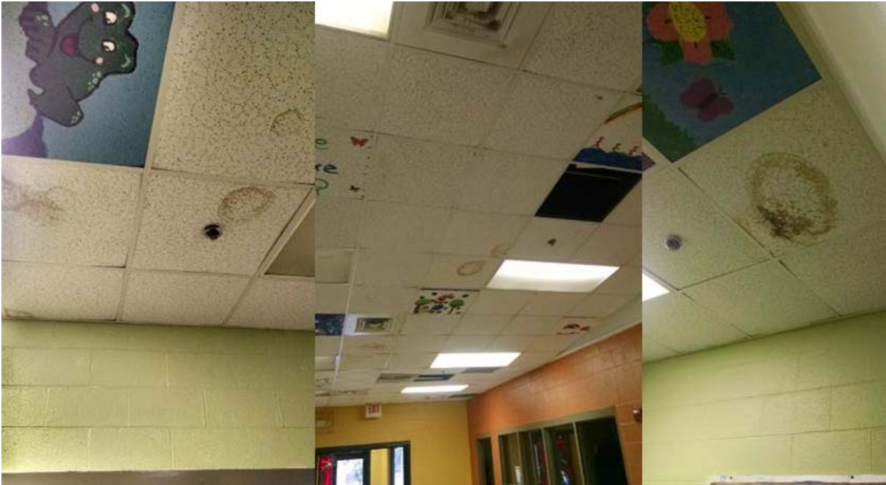
Figure 39: Moisture laden air caused numerous ceiling tile failures due to overhead plenum space connection with mechanical room louvered doors (YAC4). [Barcik photos]
