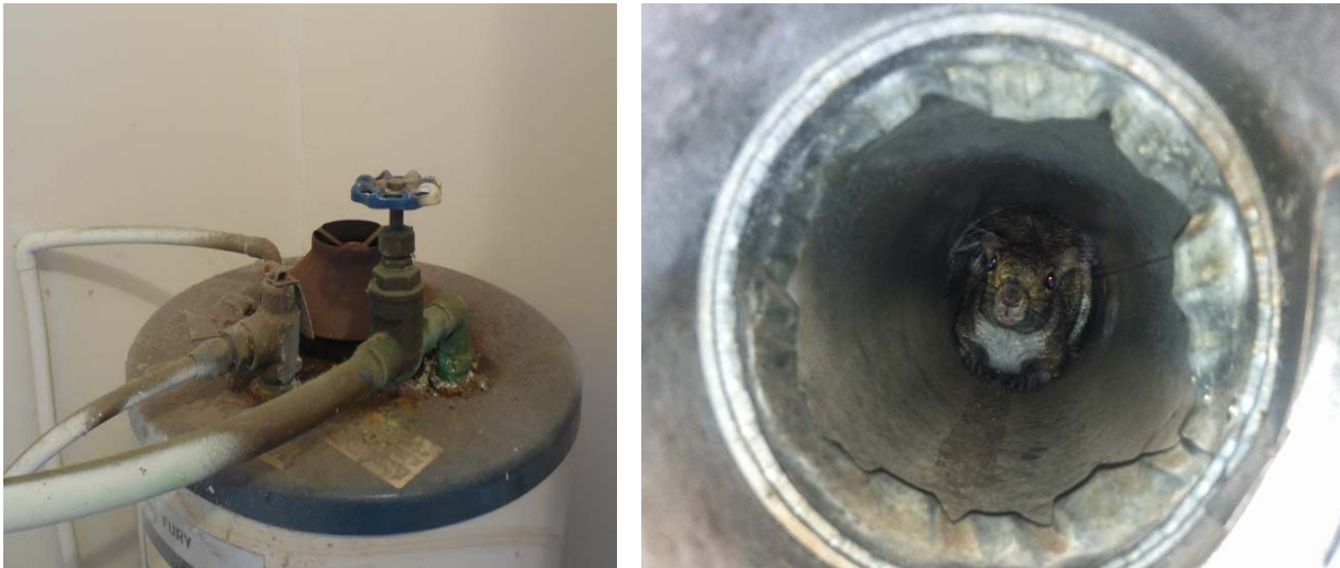
Figure 30: (Left), Should the missing flue pipe be corrected before air-sealing is conducted?! (Right), Does the squirrel in the flue pipe read disclaimers?! [D. Coffey photo (left), J. Apicella photo (right)]
