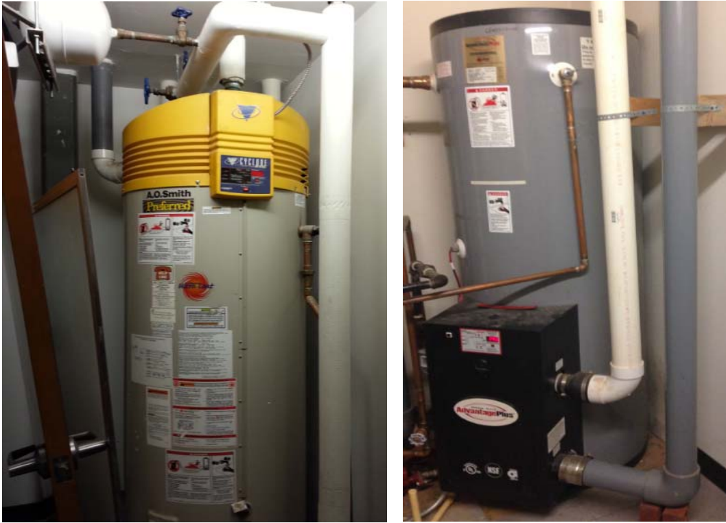
Figure 7: High Efficiency 2-pipe condensing gas tank water heaters - do not use the surrounding air for combustion air and contain no standing pilot (Fire1, Day Care) [Barcik photos]
