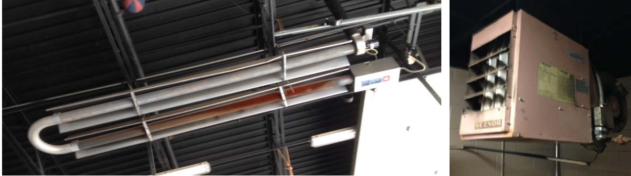
Figure 13: It is typically more efficient to use surface-warming radiant heaters in high bay applications (left, Fire1) versus hanging space heaters that attempt to heat the large volume of air (right, Fire4) [Barcik photos]
