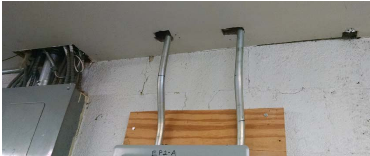
Figure 33: Currently, this closet's combustion air comes from leaks to the vented attic – this should be sealed off if the roofline is foamed and then have combustion air provided from the exterior (YAC3). [Barcik photo]
