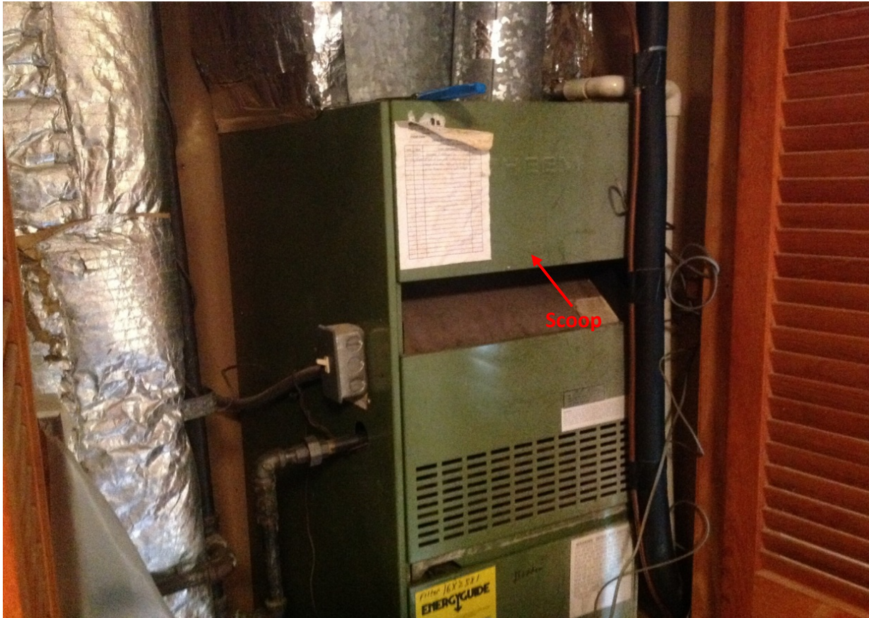
Figure 1: 60-70% furnace with louvered door for combustion air [Barcik photo]
