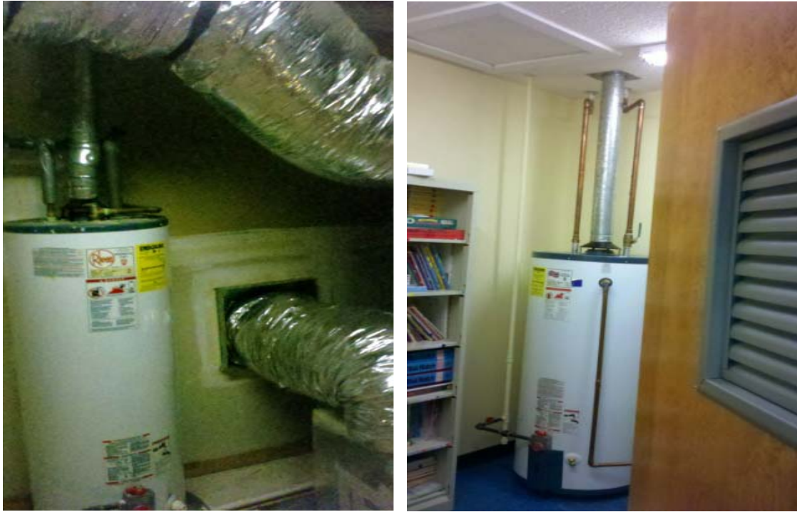
Figure 31: Small standard gas water heater in vented attic mechanical room (Early Childhood Care center, left). Large standard gas water heater in internal closet (Early Childhood Care center, right). [Barcik photos]
