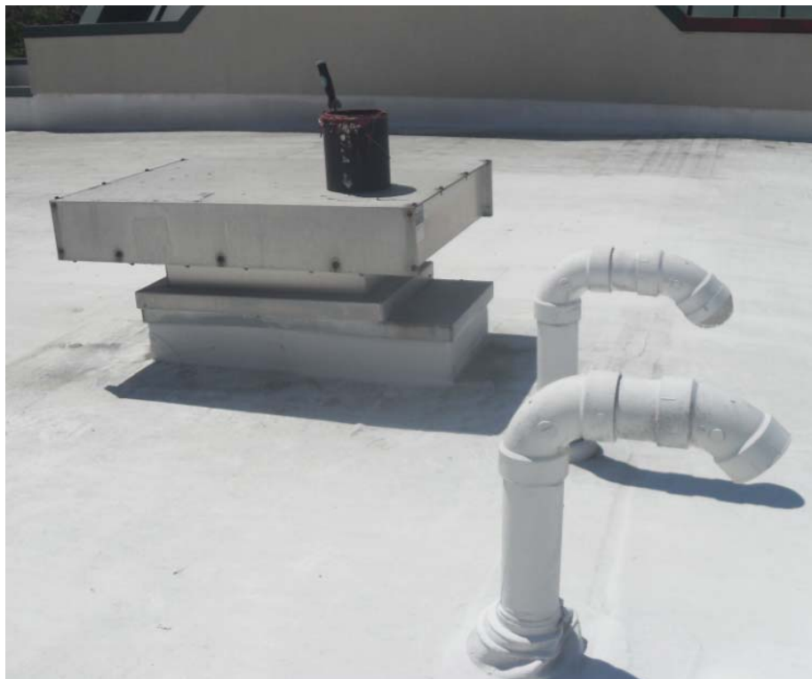
Figure 19: Paint can sits atop rooftop inlet for High-Low vents. PVC air intake and exhaust for installed condensing gas tank. (Fire1) [Barcik photo]
