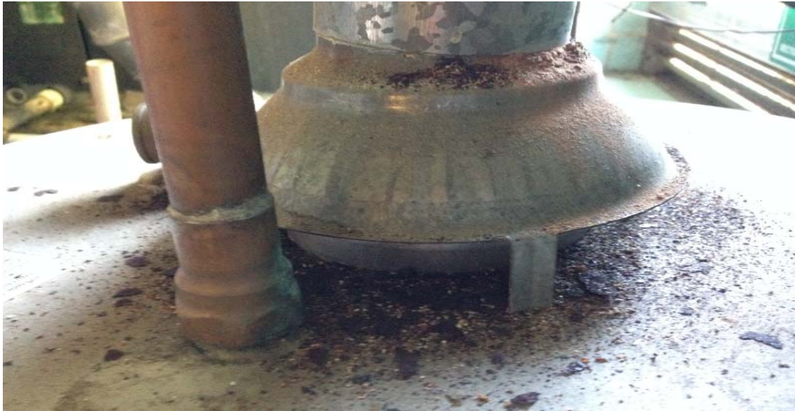
Figure 25: Corrosion on water heater draft diverter caused by condensation due to poorly drafted flue (Fire2). [Barcik photo]
