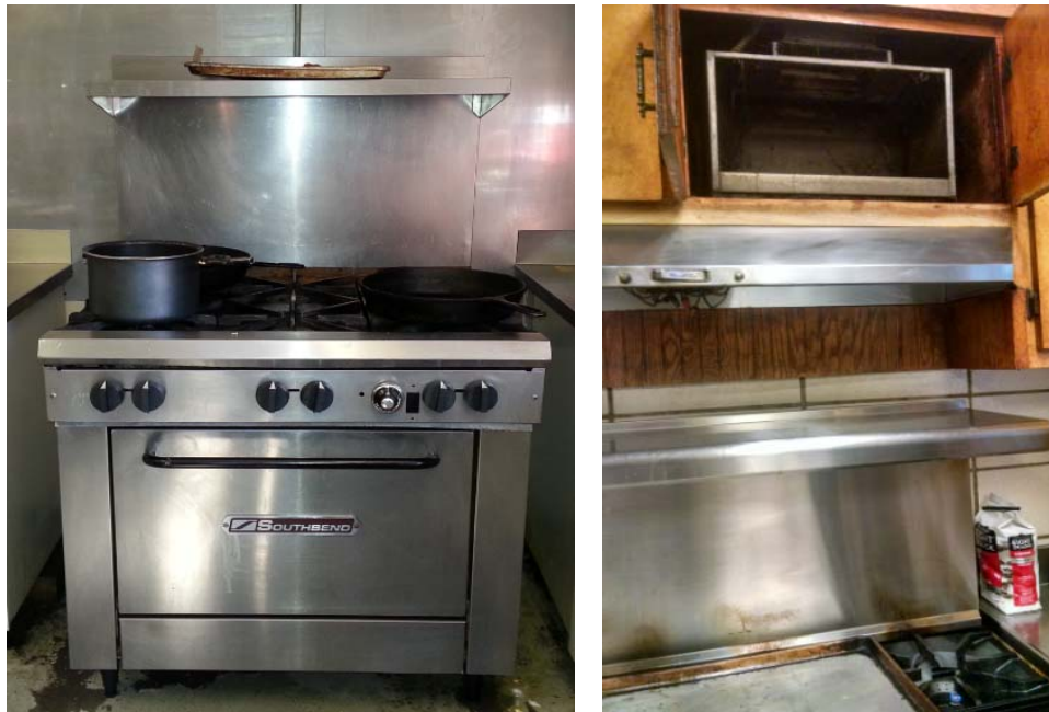
Figure 10: Always hot - Gas cooktop with pilots and no functioning exhaust hood (left), Missing fan and hood mechanism (right) (Fire1) [Barcik photos]
