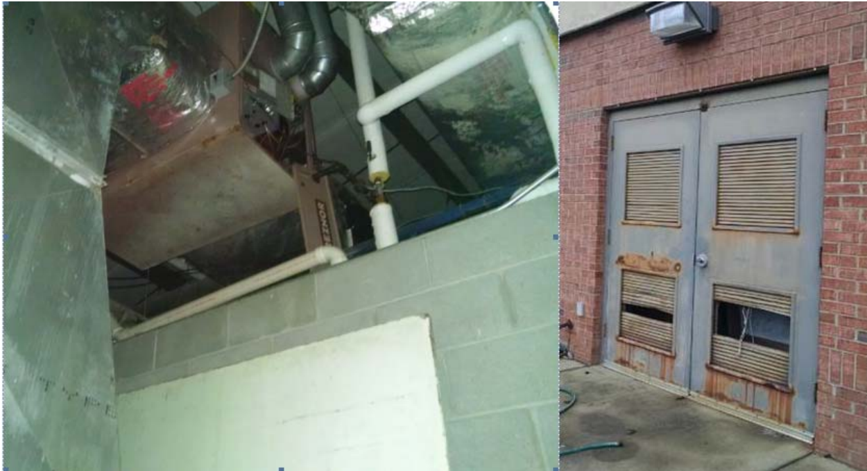
Figure 38: (Left), Furnace in highly vented mechanical room fully connects to the rest of building due to connected overhead plenum space (YAC4). (Right), Mechanical room louvered doors (YAC4). [Barcik photos]
