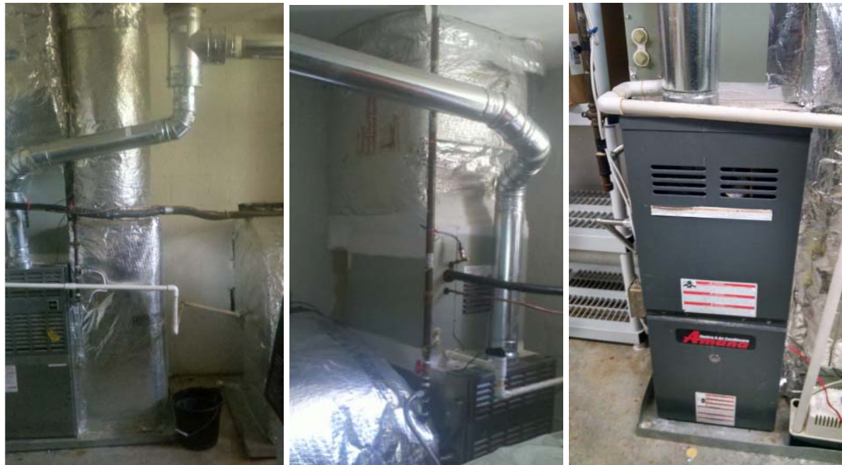
Figure 34: Three standard 80% furnaces that will require separate combustion air be provided to them if the roofline is foamed (YAC3). [Barcik photo]
