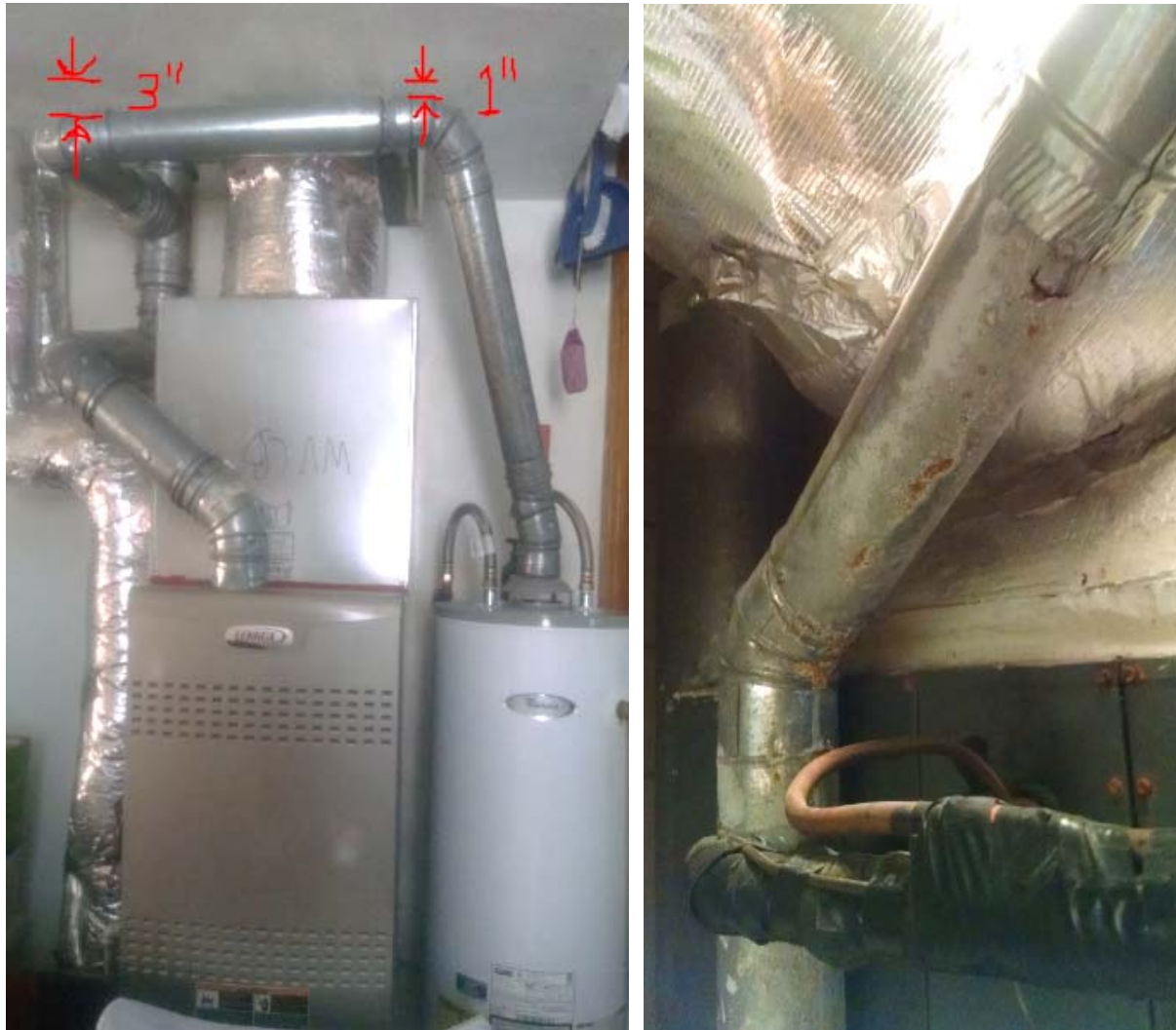
Figure 27: Oops! Water heater flue pipe drops 2" in connecting to the shared flue (Virginia1). Corrosion caused by condensation due to poorly drafted flue (Fire2). [Barcik photos]
