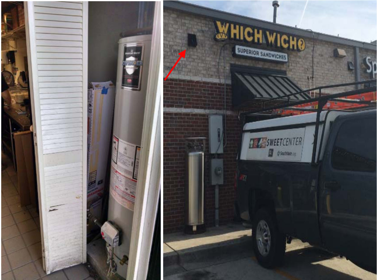
Figure 37: (Left), Standard gas water heater in closet with louvered door (Restaurant1). (Right), Note unused wall penetration that could be ducted to provide air to the combustion closet (Restaurant1). [Barcik photos]
