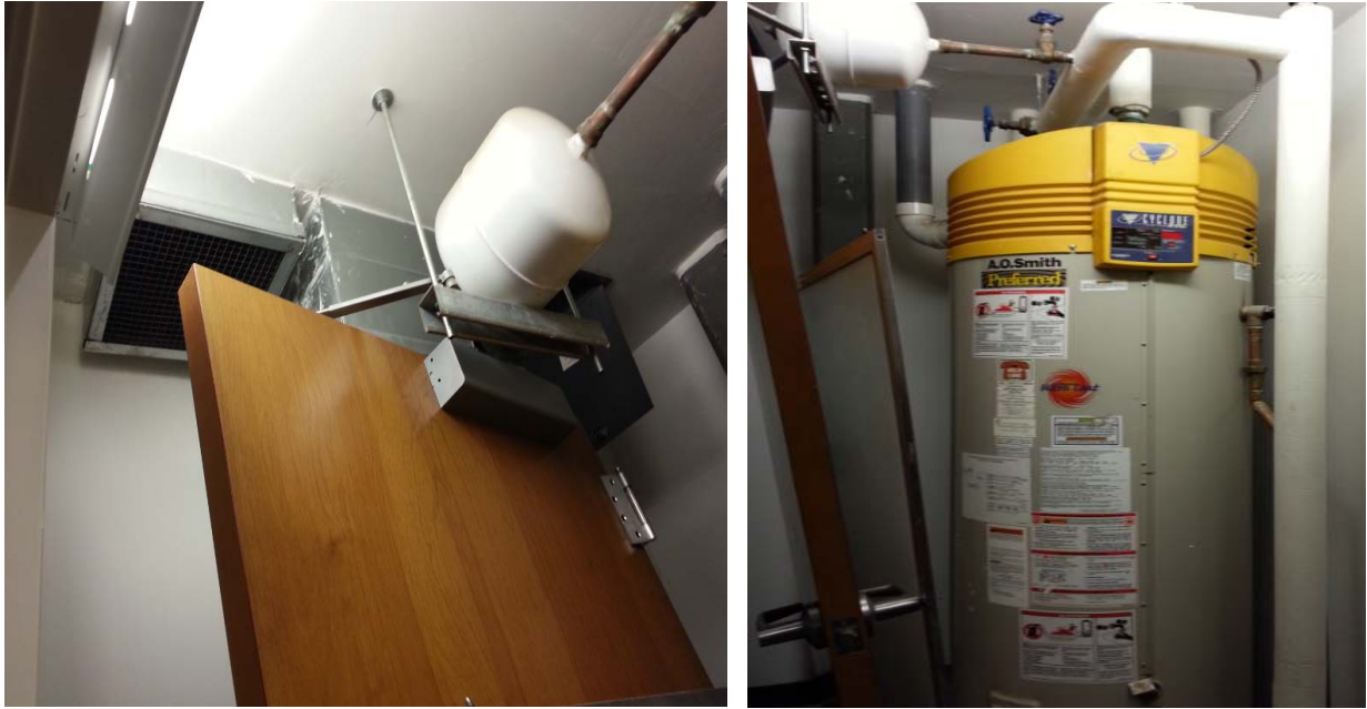
Figure 20: Interior closet view of High-Low vents that should be sealed over or removed (Fire1). Condensing gas tank water heater with PVC air intake and exhaust (Fire1) [Barcik photos]
