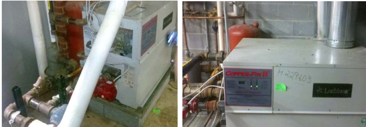
Figure 9: Two views of a standard boiler and circulation pump (Youth Activity Center 2) [Barcik photo]
