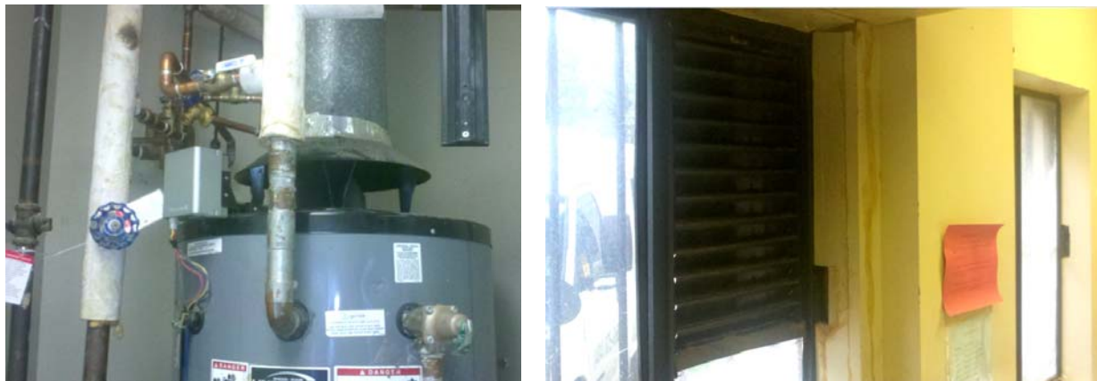
Figure 21: Atmospheric gas water heater (left) & combustion air louvers (right, Pre-school1).[Barcik photos]
