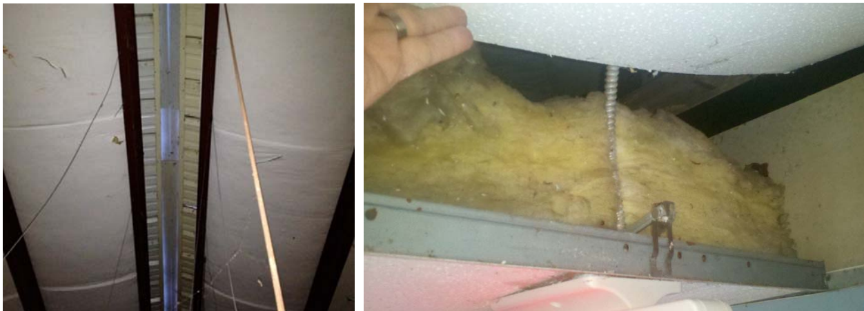
Figure 32: (Left), Ridge and soffit vents with insulation installed at roofline? Never vent under the insulation! (YAC3). (Right), a horrible detail – never put insulation batts on drop ceiling tiles! (YAC3). [Barcik photos]
