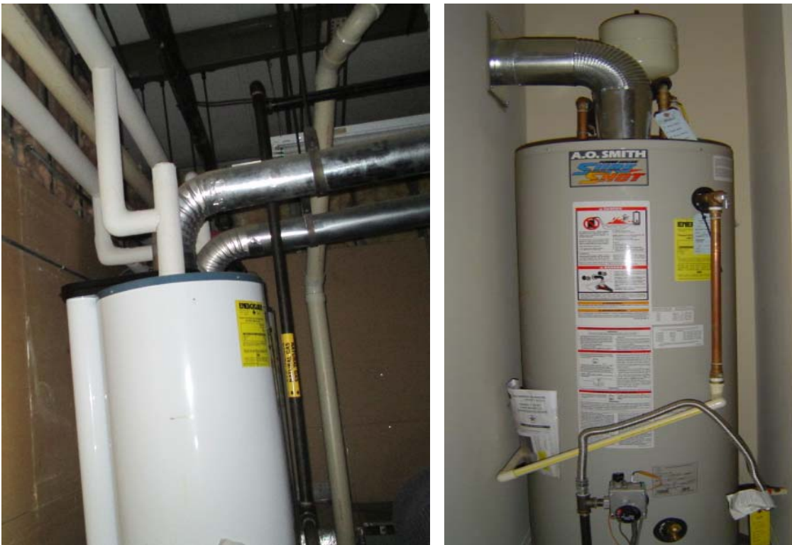
Figure 5: Direct vent gas water heaters – do not use air around them for combustion air (Youth Activity Center 1, garage demo) [Barcik photos]
