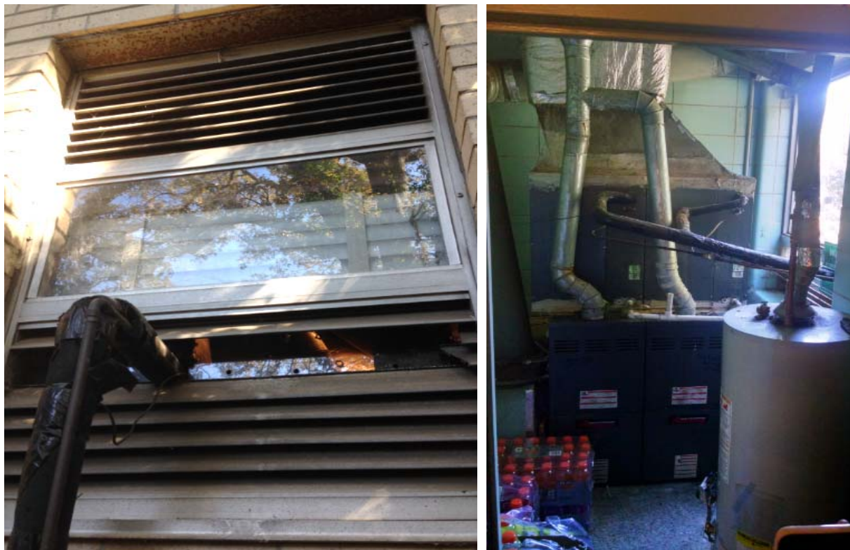
Figure 23: Occupants added plexi-glass to seal off outdoor combustion air louvers because of cold air drafts since there were also louvers connecting to the conditioned space (left, Fire2). Common-vented appliances are often easier to backdraft due to their large-sized flue pipes (right, Fire2) [Barcik photo]
