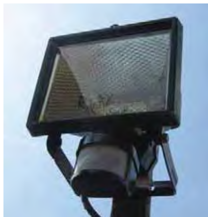
Motion sensor on pole-mounted 150 W halogen floodlight.
