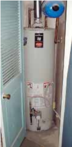
This combustion closet draws air through a louvered door, this is not recommended.
