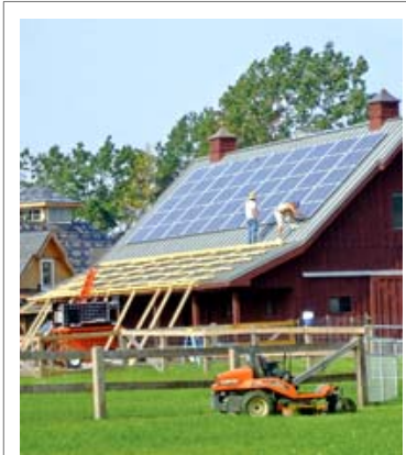
Courtesy of Sue Leone — Solar panels on the Leones' barn store energy and send excess back into New York's power grid.
